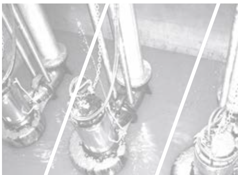
Wastewater Transport and Treatment
