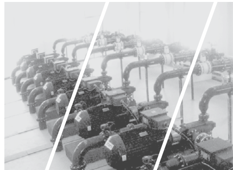
Boosting and Distribution of surface water
